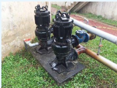
CNT (Dry Pit Pump)
