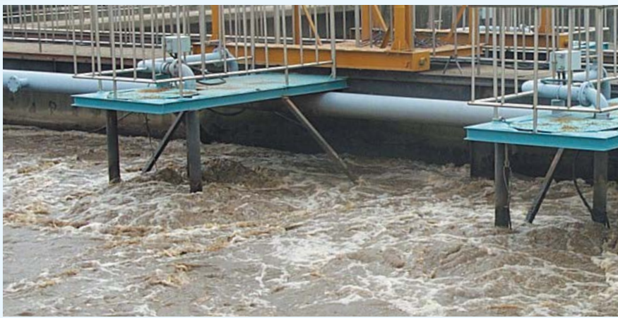
Submersible aerator "SJ" is now in operation
