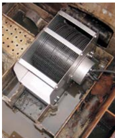
Site: Onsite wastewater treatment system
