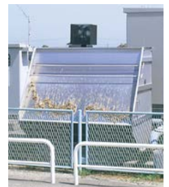
Site: Pump station (River water intake)
