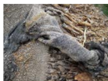
Grinder pump clogging with rags
